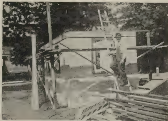
Concrete walls completed and forms removed. In many cases walls would be left as shown. In this instance they were given a dash finish. Note use of scaffold brackets
